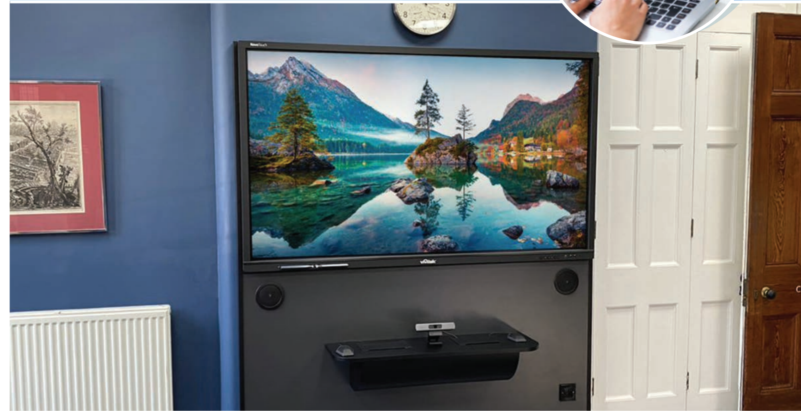
Above: Wall-mounted video conferencing solution installed at Girton College Cambridge College
